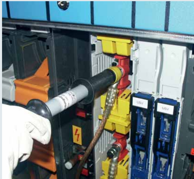
Attaching a partly insulated earthing and short-circuiting device using an earthing handle of type TI
